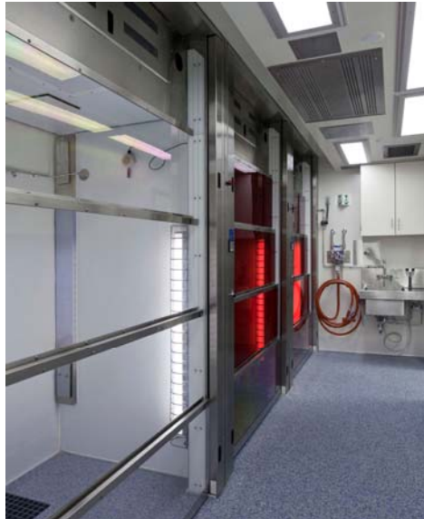
Individual housing cubicles accommodate reverse light cycle housing and flexibility.
